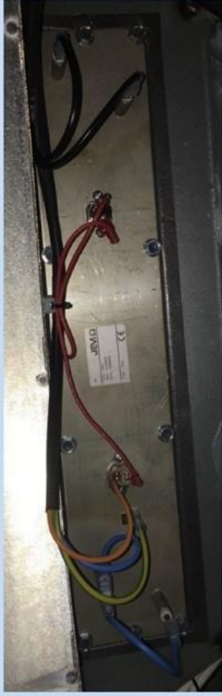
Electric heater foto
